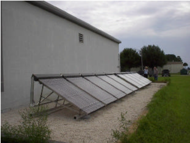
Figure 8: The Thermomax tubes at the Kennedy Space Station in Florida supplies 53,000 BTUH (200 + °F) to drive desiccant cooling units.
