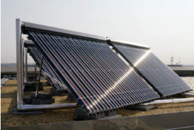
Figure 7: The Pentagon evacuated heat pipe solar system is the largest solar thermal system of its type in North America with a rated peak thermal output of 75.6 kW.
