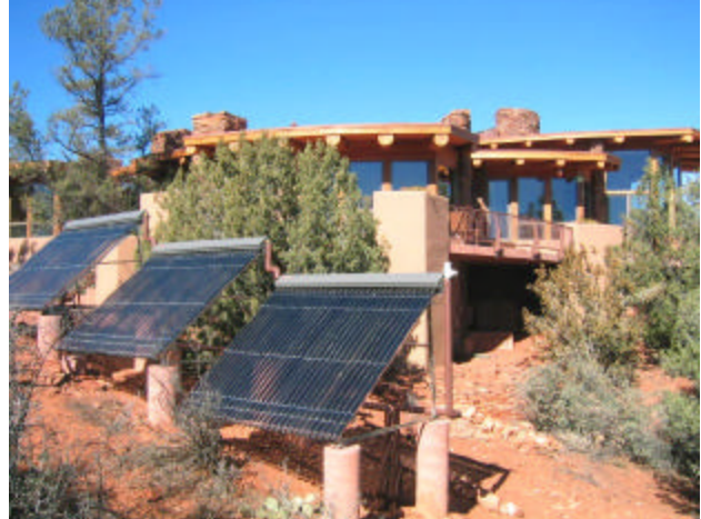
Figure 9: The 6.3 kW solar thermal energy (system shown above) in Sedona, Arizona, is the space heating primer source.
