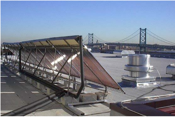
Figure 1. Photograph of the solar array on the southwest riser of the building recirculation loop on the Mid-Atlantic Social Security Center, Philadelphia, PA; another array on the northeast riser is identical in size and orientation.
